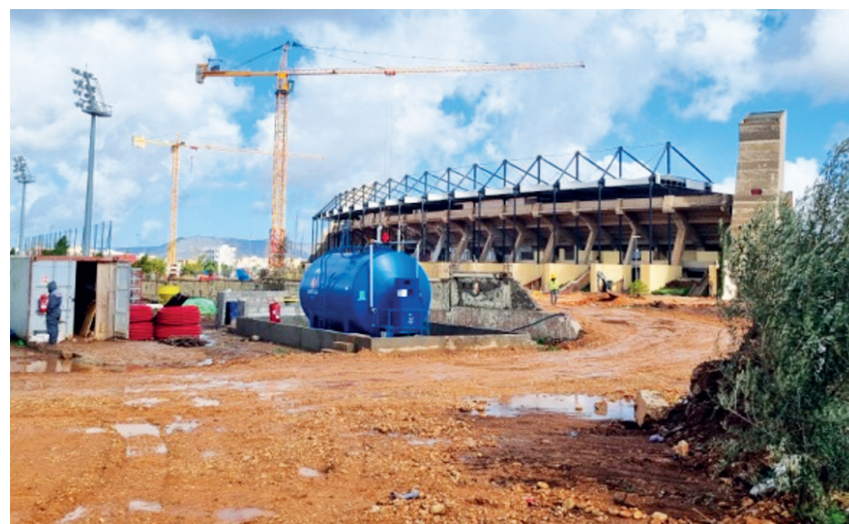
Renovation work has already begun on the Fez sports compound. The renovation project for this 45,000-seat stadium will cost 300 million DH (US 30 million) (Photo by YSA)
