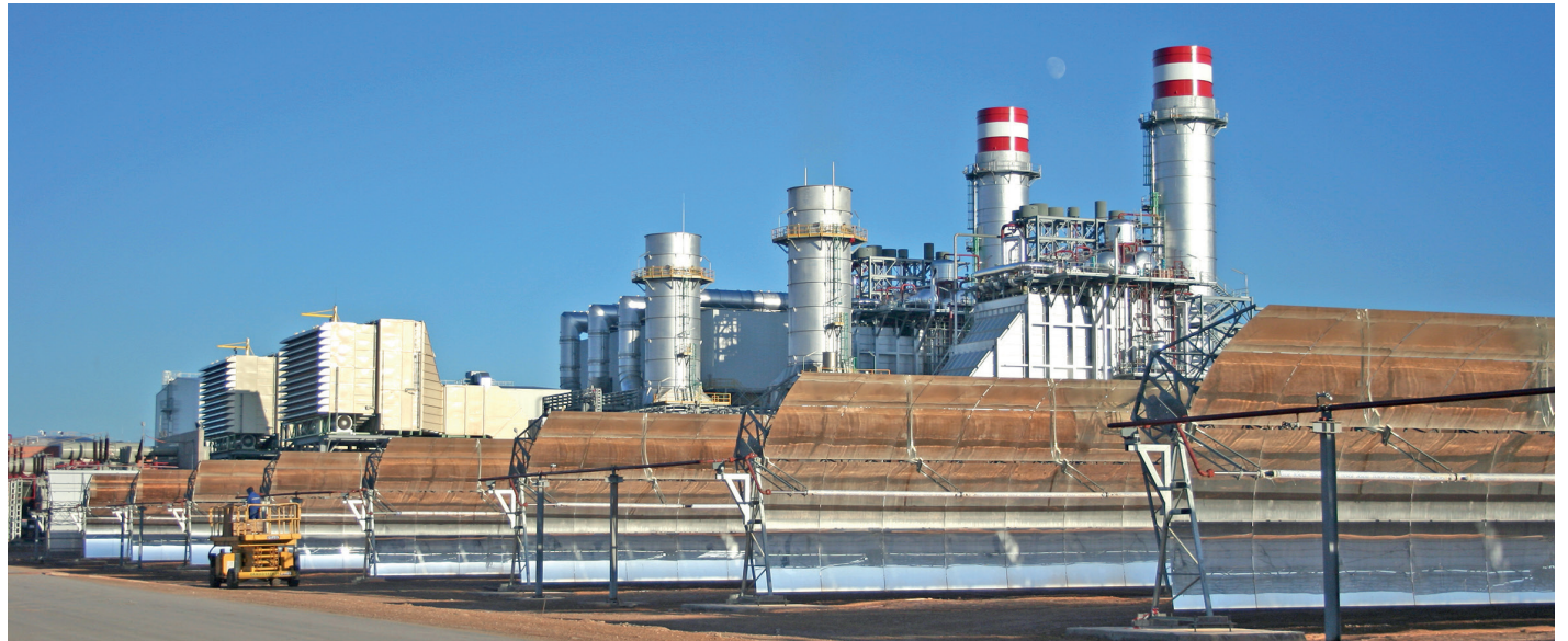
The Ain Béni Mathar plant (in the Eastern region) is located not far from Jerada, a few kilometers from the border with Algeria
